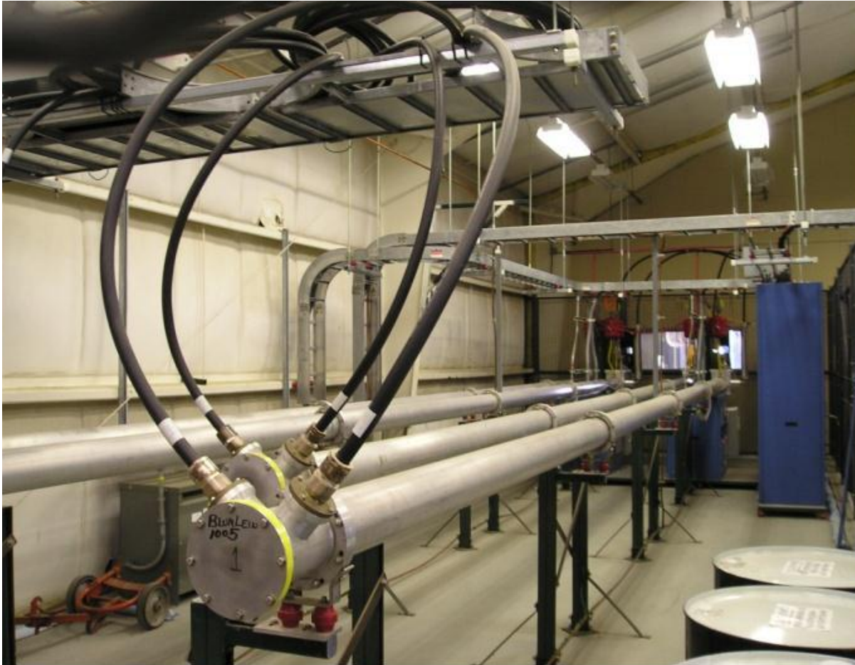
Few triaxial Blumlein generators at RHIC inflector
