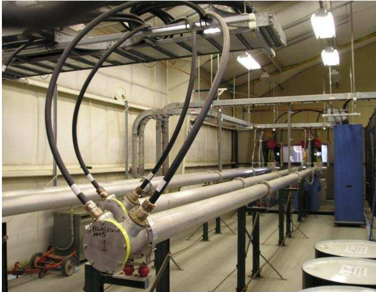
Few triaxial Blumlein generators at RHIC inflector
