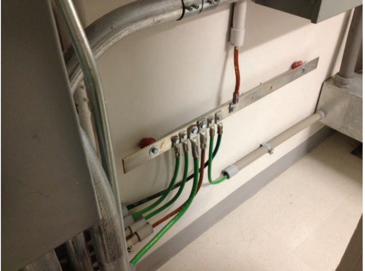
Figure 11. Photograph of detail D1 on the drawing in Figure 7 that shows how the grounds on each floor are tied together in the electric room.
