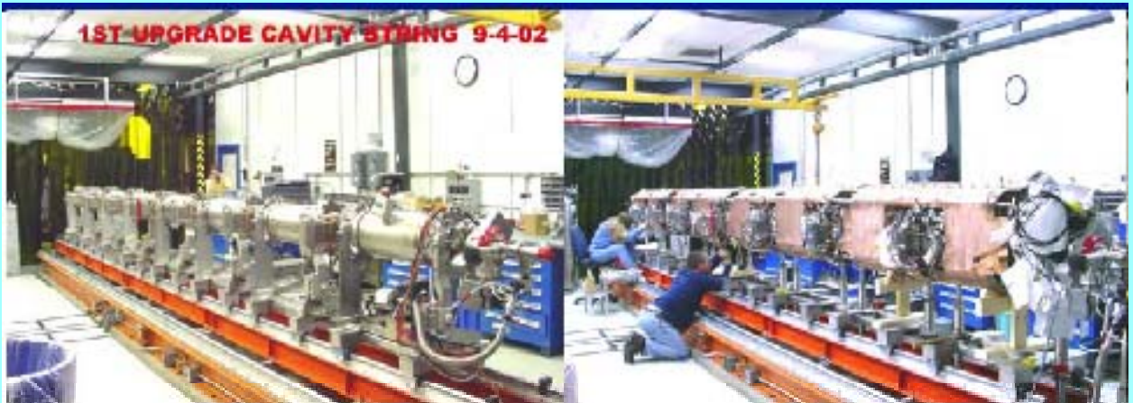
Cryomodule assembly at JLAB
