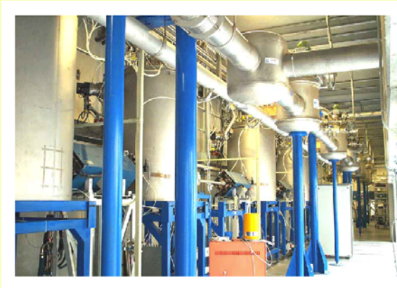
Inside ALPI at INFN Legnaro. ALPI has been in operation since 1994. 30 QWR Nb/Cu are in the beam line operating at about 4 MV/m at 7 watts dissipation. 12 Nb resonators are also in the beam line and operate at 6 MV/m with 7 watt dissipation. Typical beam time was between 3700 hours and 5000 hours from 1999 – 2000, with 25% of the time using the SC booster, since many experiments desired lower energies.
