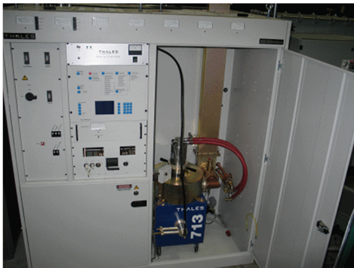
Figure 2.3.15: IOT inside the transmitter.
