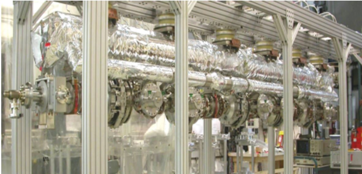
Figure 2.4.34: Beamline string hung from the HGRP for the ERL Injector.
