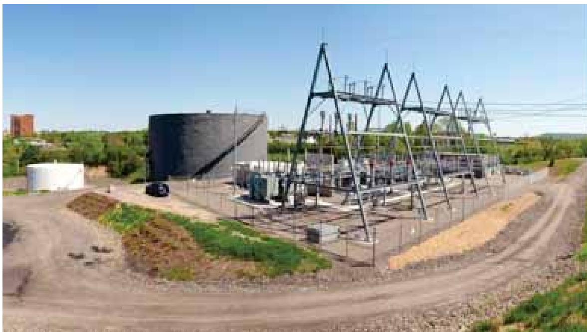
Figure 4.4.2: Maple Avenue substation.
