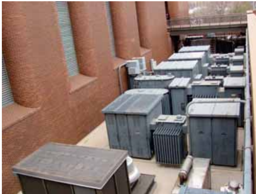
Figure 4.4.4: The Wilson Lab fourth-floor transformer pad
