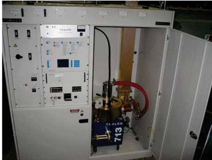
Figure 2.3.15: IOT inside the transmitter.
