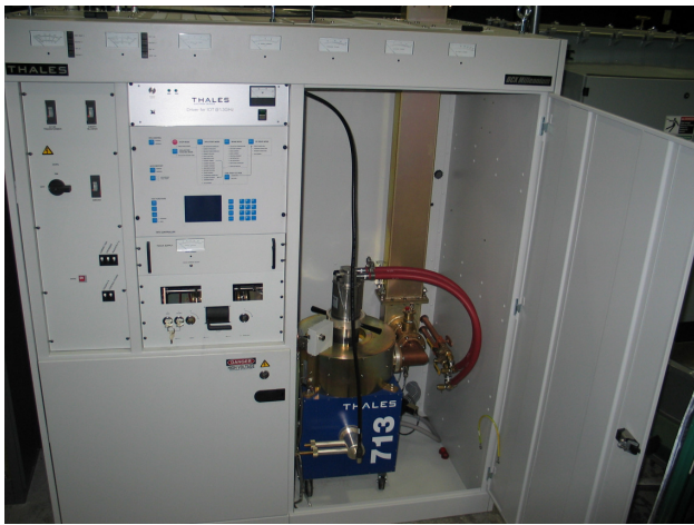
Figure 3: TH 713 IOT inside the transmitter.
