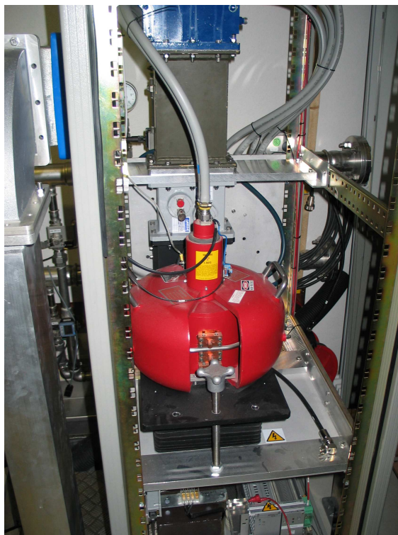
Figure 4: 10 kW CW CPI klystron inside a transmitter rack at Rossendorf.
