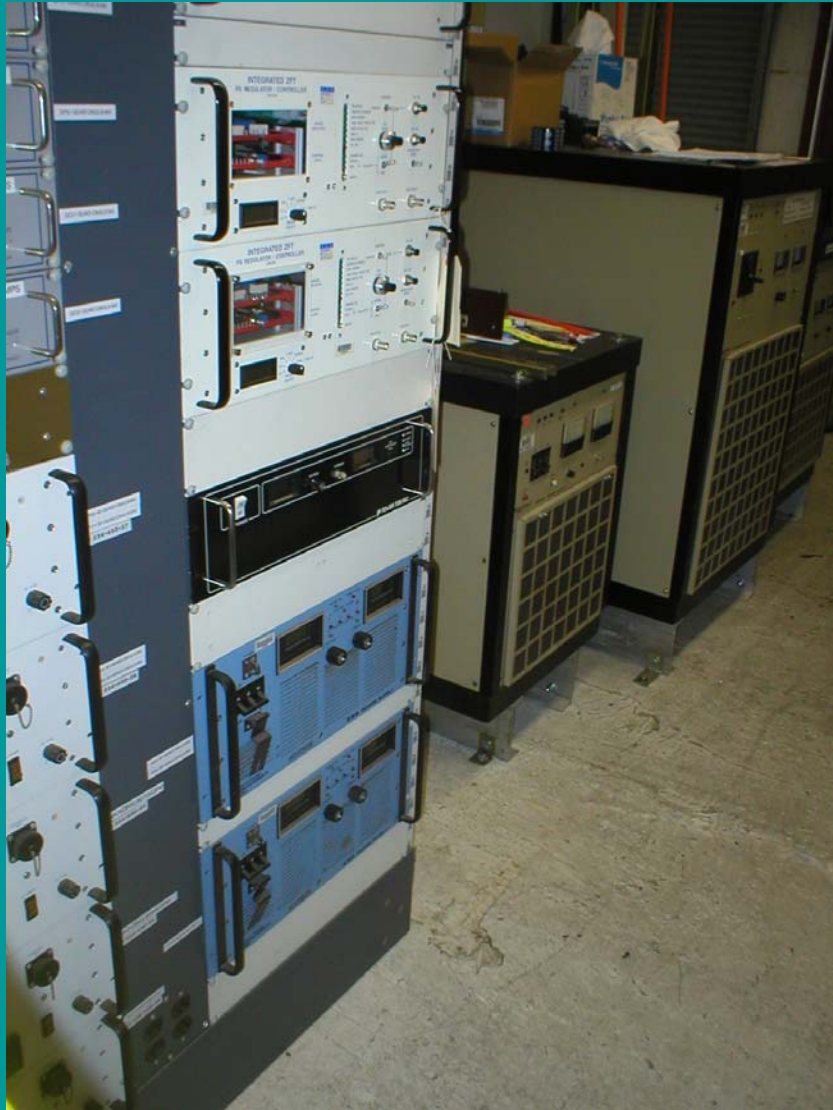
Power Supply Rack
