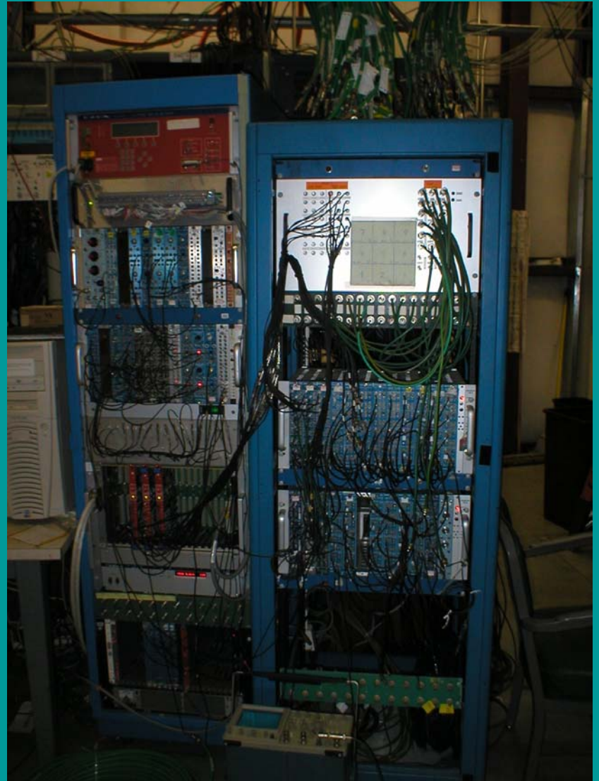
E166 Data Acquisition Rack Building 407
